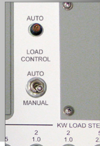
ASCO Automatic Load Control toggle switch shown on load bank control panel.
